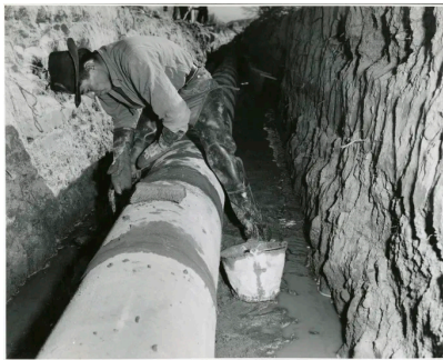
A member of a CCC-ID crew cementing the joints in a pipeline built on Santa Clara Pueblo lands for irrigation and drinking water in December, 1940. (W. J. Mead / National Archives)
